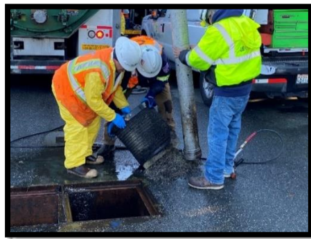
Figure 8-1. A crew replaces a stormwater filter in a catch basin at near Guemes Island Ferry Terminal
